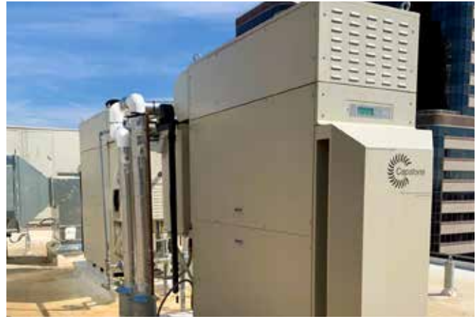
Two Capstone C65 ICHP microturbines ensure high reliability while also benefiting the environment.
