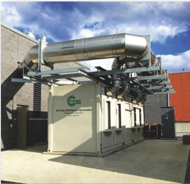
A Capstone C800 microturbine operating in a CCHP application producing 800kW of clean and reliable power for the PSECU data center UPS, located in Harrisburg, Pennsylvania. Source: Capstone Turbine Corporation
