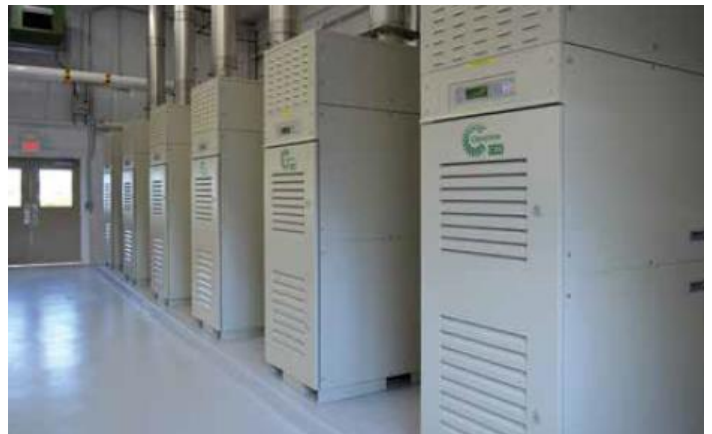
Natural gas fuels six Capstone C65 Integrated CHP microturbines that produce 390kW of clean and reliable power as well as thermal energy for the Viking Yacht Company, located in New Gretna, New Jersey. Source: Capstone Turbine Corporation.
