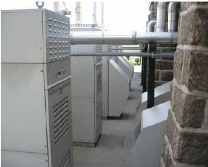
Capstone microturbines generate electricity and heating at Masonic Village, a 1,400-acre complex serving more than 1,700 residents since 1910, located in Elizabethtown, Pennsylvania. Source: Capstone Turbine Corporation
