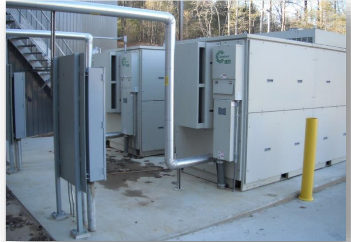
Capstone's biogas project at the Sierra Nevada Brewery site located in Mills River, North Carolina. Source: Capstone Turbine Corporation
