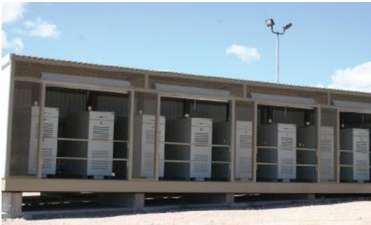
Fifteen 65 kW Capstone microturbines running on propane provide primary power for a booster station on an oil pipeline at Ramon Station in New Mexico, US.
