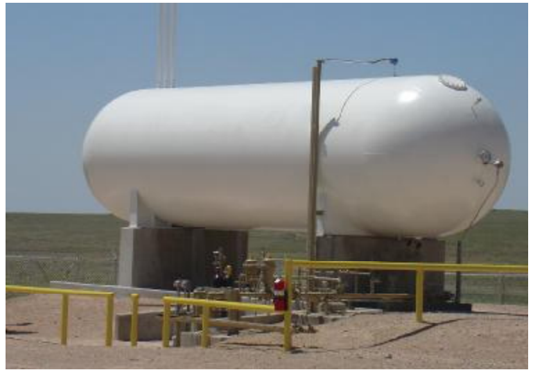
Propane tank fueling microturbines at Ramon Station.
