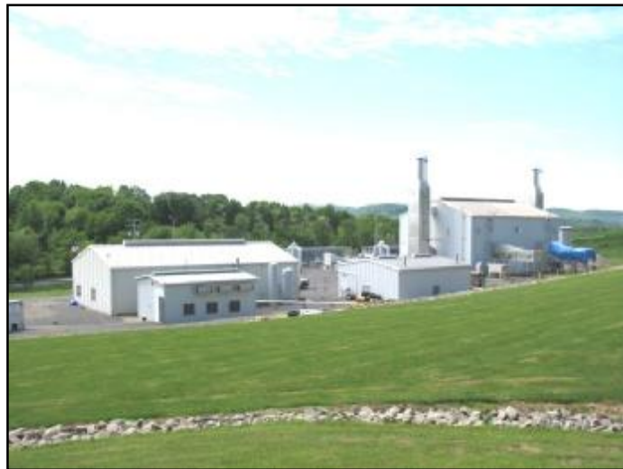
Dominion Transmission’s Crayne Compression Station in Pennsylvania, where three Capstone C65-ICHP MicroTurbines™ provide all electricity and heat for the 5-acre site.
