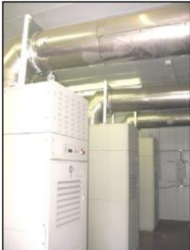
Three Capstone C65-ICHP microturbines operate on the pipeline natural gas that's pumped through Crayne Station. Heat exchangers on the top of each microturbine capture waste heat used in the decompression process.
